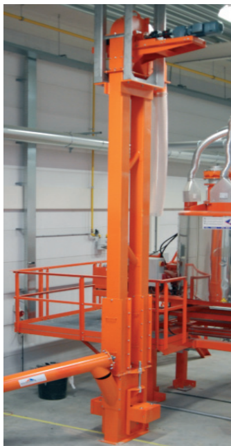
Elevator loaded by weighed screw conveyor
